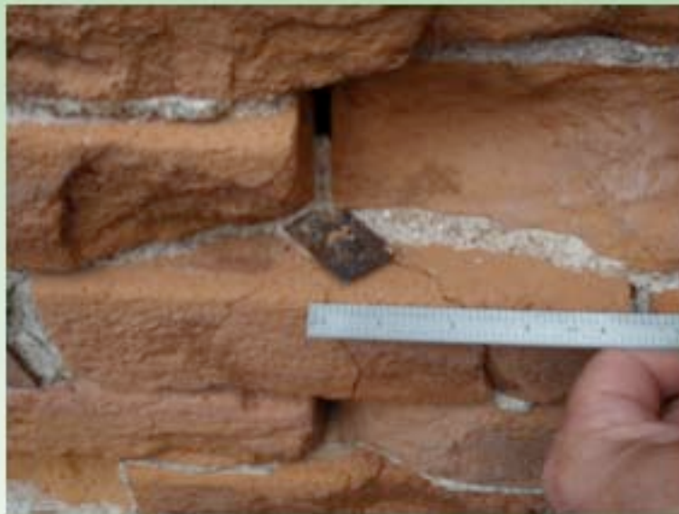
Moderate corrosion Corrosion-related expansion: brick damage at one location
