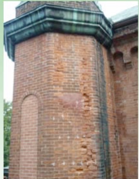
Other locations: faulty tie installation
